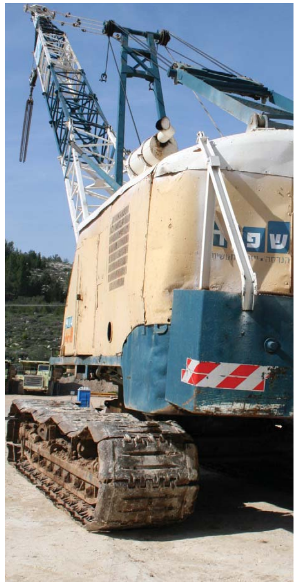
Machinery with the logo of Shapir Engineering, in the construction site for Section C, January 2010
