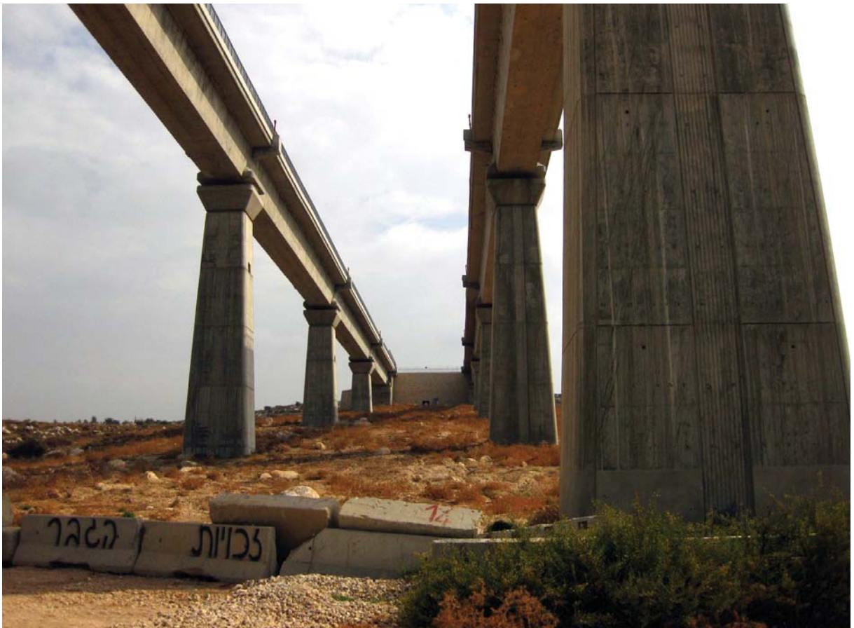
The east end of Bridge 6, at the point of entry into Tunnel 1, deep inside the Latrun Enclave
