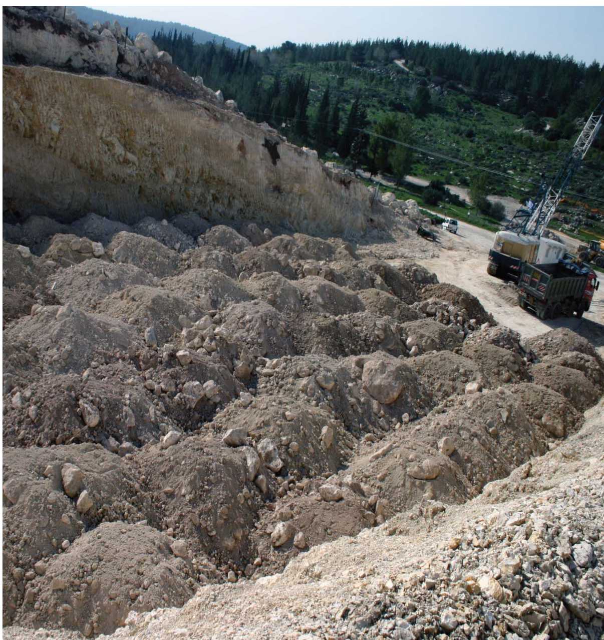
Preparation digging for Tunnel 2 in the main logistics base for Section C, Sha'ar Hagay, January 2010.
