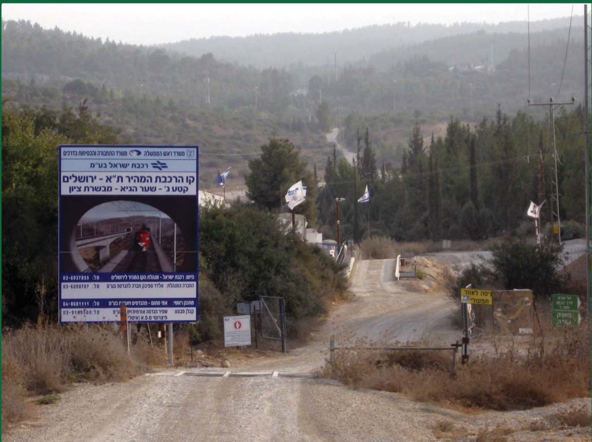
The entrance to the main logistics base for the construction of Section C of the railway, October 2010
